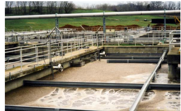
Water Treatment Plant FIMS Usage Code: 5129
