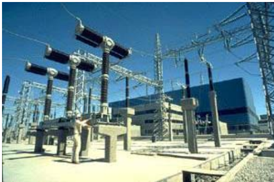
Electrical Substation FIM Usage Code: 8979
